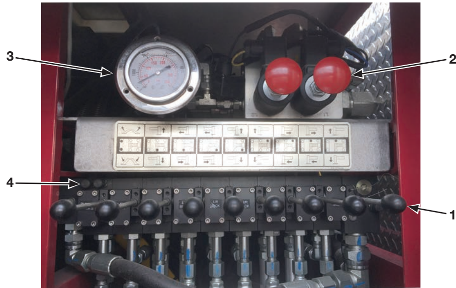
Figure 3-24. Direct Hydraulic Beam and Jack Controls
