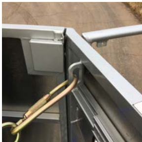
Figure 4-8. Approved Fall Protection Anchor Point
