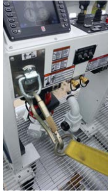
Figure 4-11. Approved Fall Protection Anchor Point
