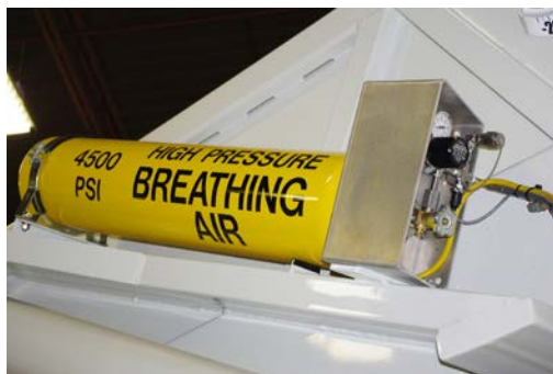
Figure 3-19. Breathing Air System High-Pressure Cylinder
