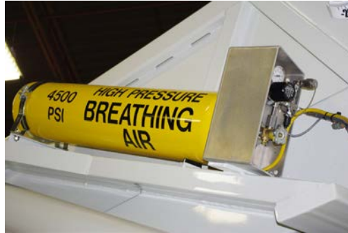
Figure 3-20. Breathing Air System High-Pressure Cylinder
