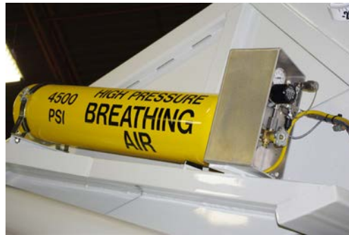
Figure 3-20. Breathing air system high-pressure cylinder
