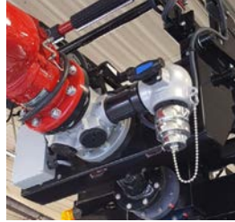
Figure 4-16. Aerial Standpipe Connection
