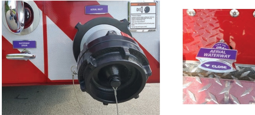
Figure 3-24. Waterway Drain and Aerial Inlet
