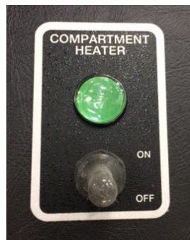
Figure 3-6. Pump Compartment Heater Control
