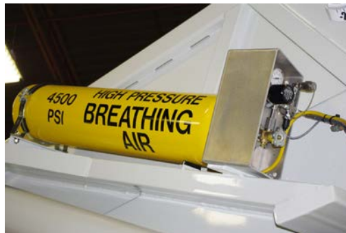
Figure 3-27. Breathing Air System High-Pressure Cylinder
