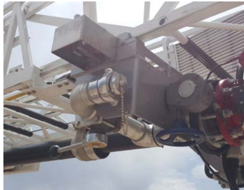
Figure 4-13. Aerial Standpipe Connection
