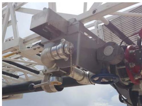
Figure 4-14. Aerial Standpipe Connection
